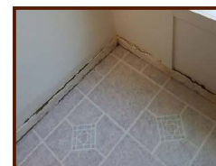
Minor water damage
