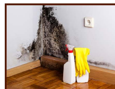
Moderate mold damage
