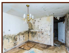
Home with major damage
