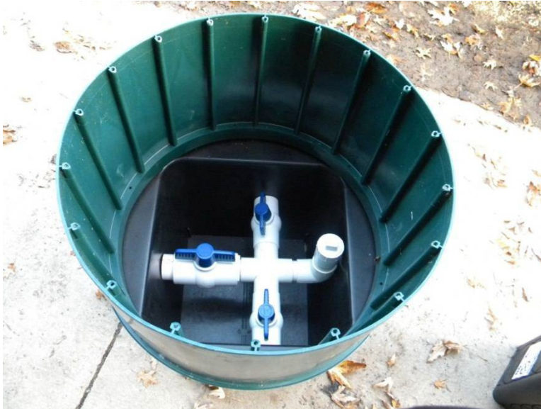
Figure 7. Service box within the manifold line
